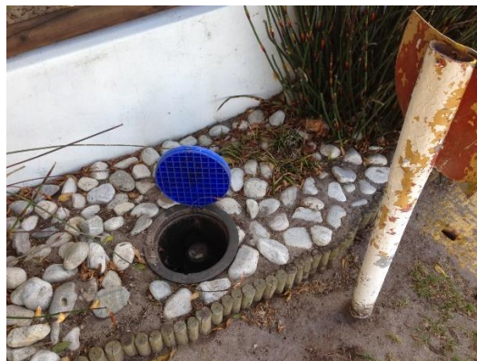
Figure 20: Location of Water Supply Stopcock
