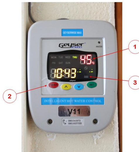
Figure 16: Solar Geyser Control Panel
